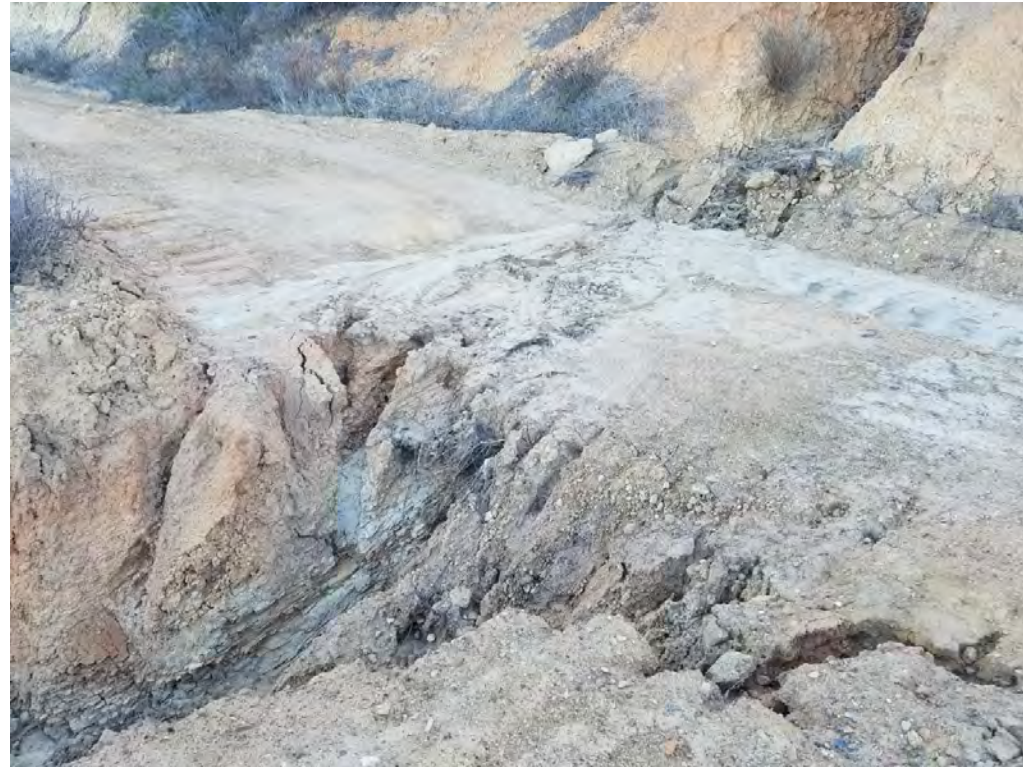
Photograph 1: Close-up view of access road erosion recommended for repair. Photo taken November 3, 2021.
