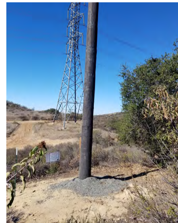
Photograph 4: New or newly replaced SCE pole on OCTA property. Photo taken November 3, 2021.
