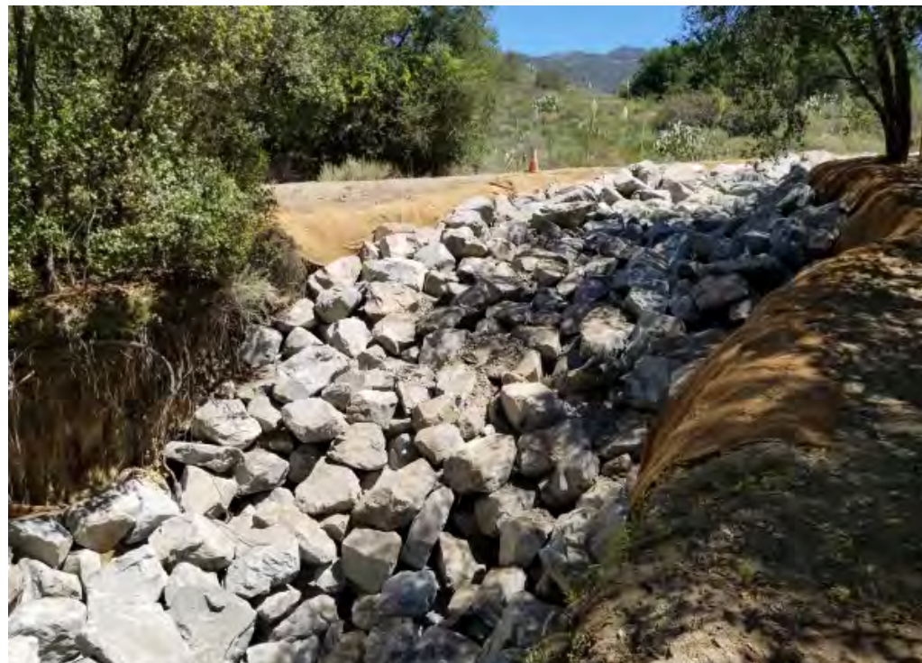
Photograph 11: View facing east of gully erosional repair area post-installation. Photo taken May 25, 2021.
