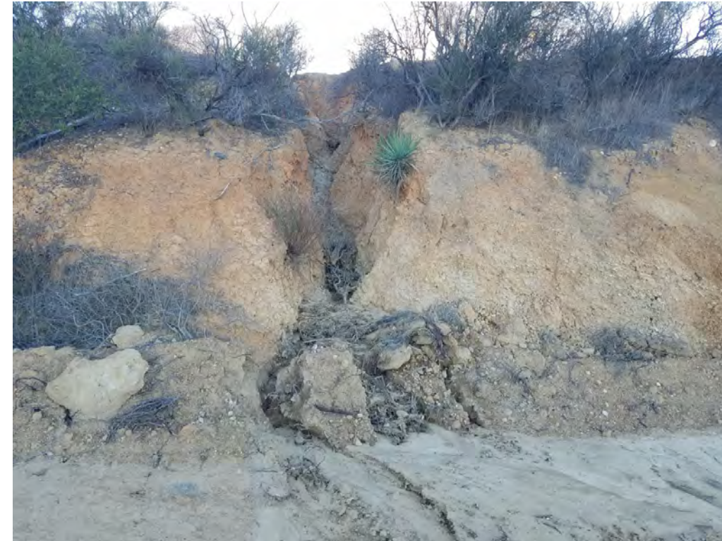
Photograph 2: View of erosion facing west. Photo taken November 3, 2021.
