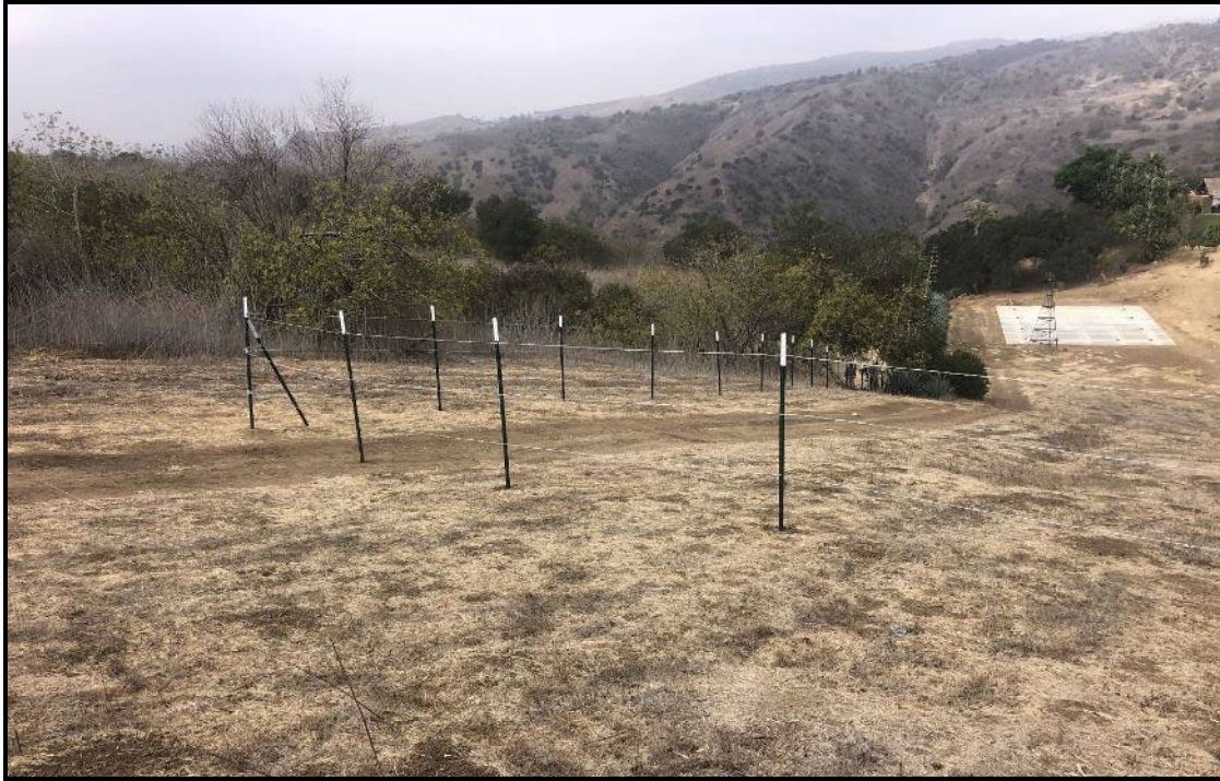
PHOTOGRAPH 38 New Fence Line at Northern Edge of Property, Following Installation, Eagle Ridge Preserve, October 2021
