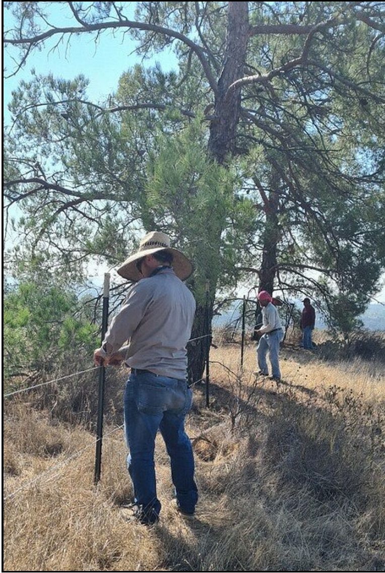
PHOTOGRAPH 9 Repairs to Damaged Fence in Northern Section of Trabuco Rose Preserve, October 2022
