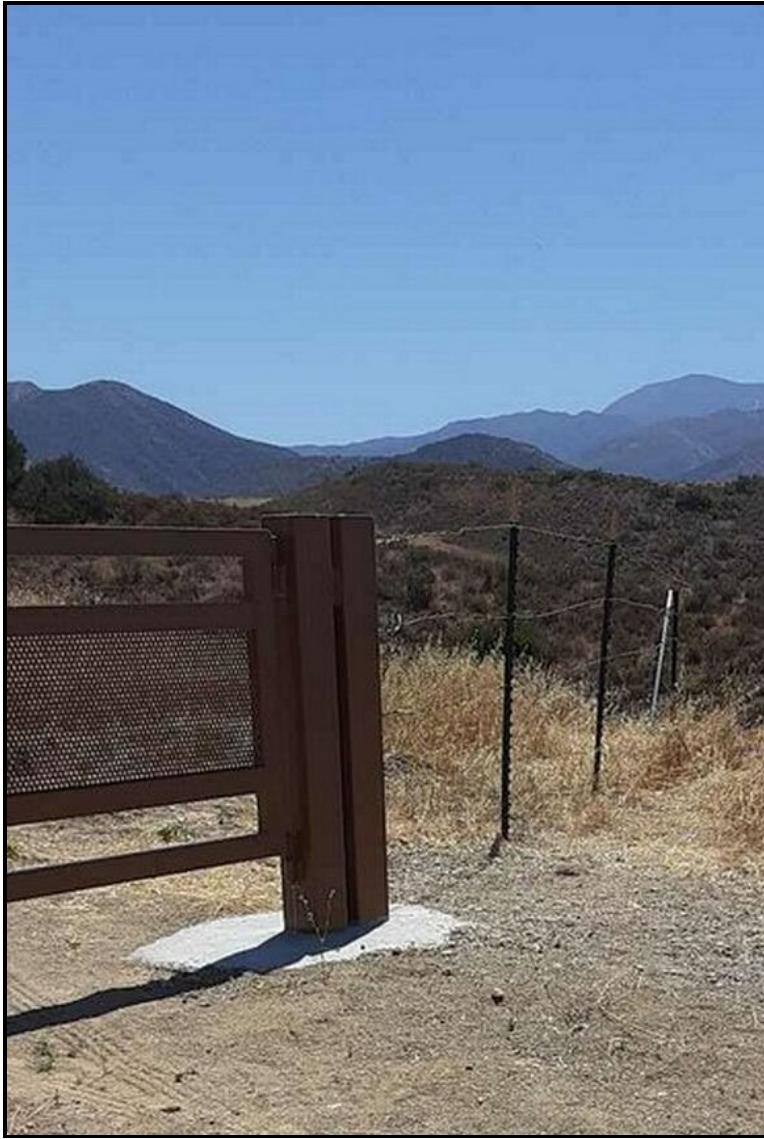
PHOTOGRAPH 20 Installation of New Fence Line, Connected to New Gate at Silverado Chaparral Preserve, June 2022
