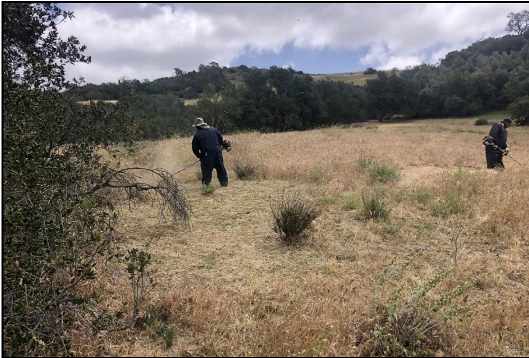
PHOTOGRAPH 13 Vegetation Control with Line Trimmers within a Fuel Modification Zone at Live Oak Creek Preserve, May 2022
