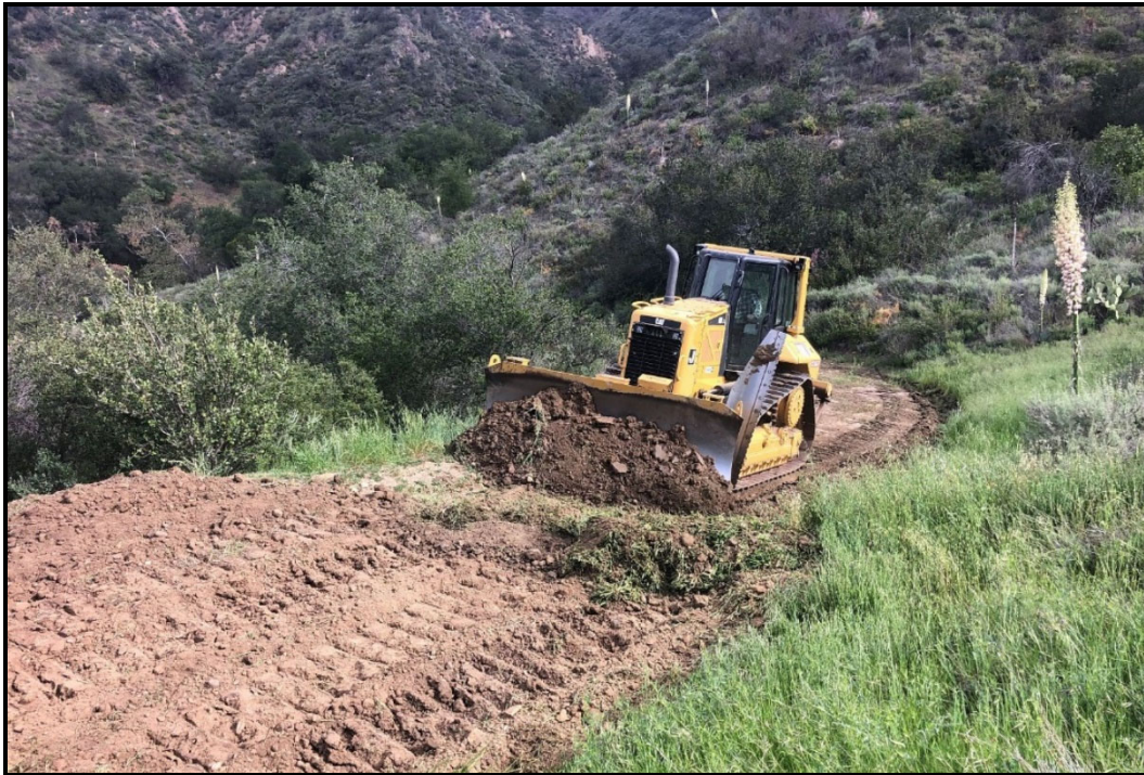
PHOTOGRAPH 4 Recontouring of Fire Roads with Heavy Equipment to Fix Erosion at Trabuco Rose Preserve, April 2022
