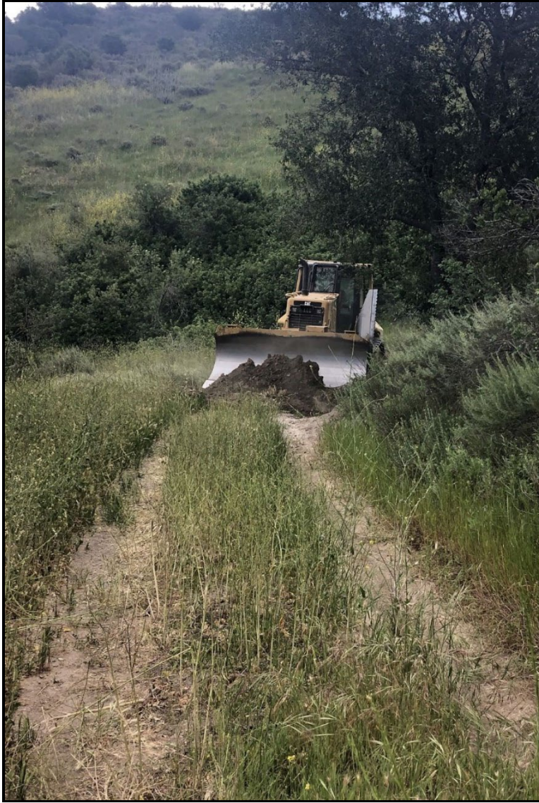
PHOTOGRAPH 12 Recontouring of Fire Road with Heavy Equipment to Fix Erosion at Live Oak Creek Preserve, April 2022
