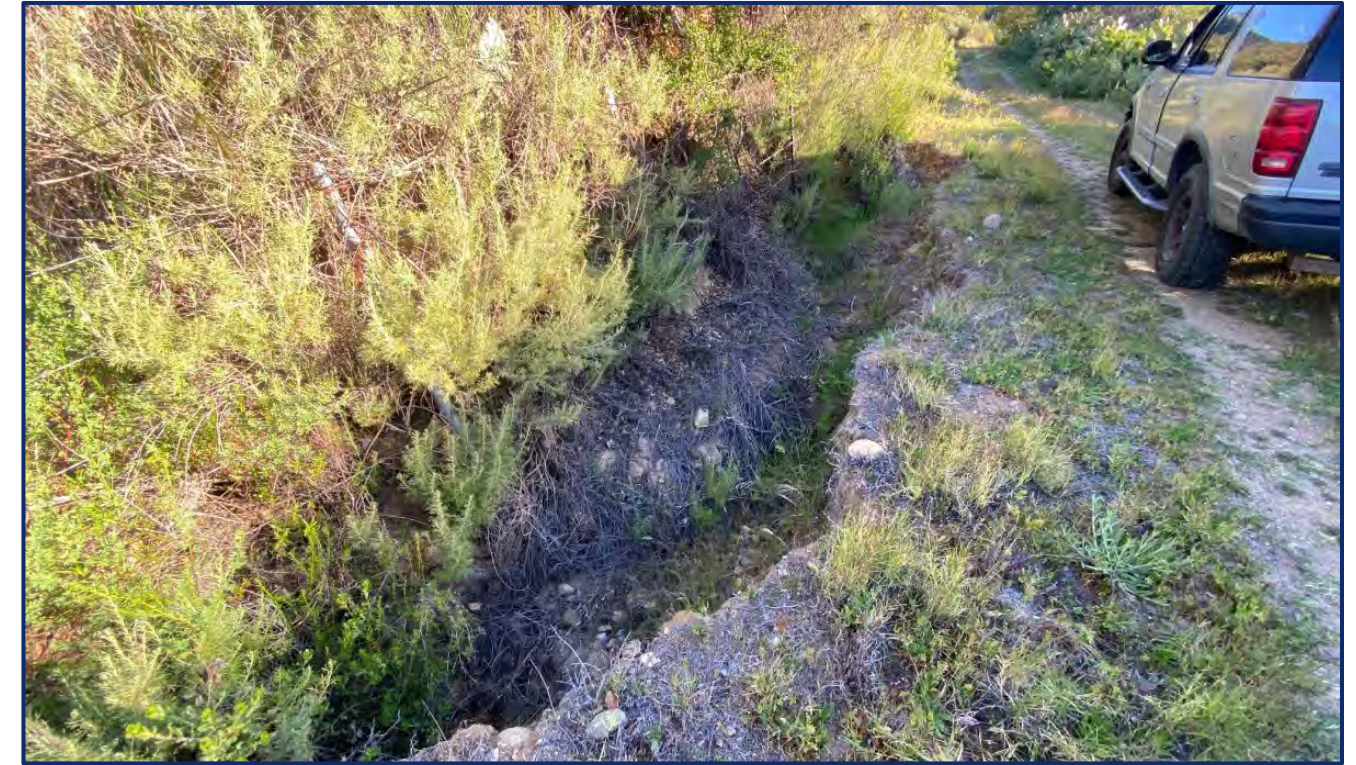
Photograph 2: View of erosion along main access road. Photo taken March 22, 2022.
