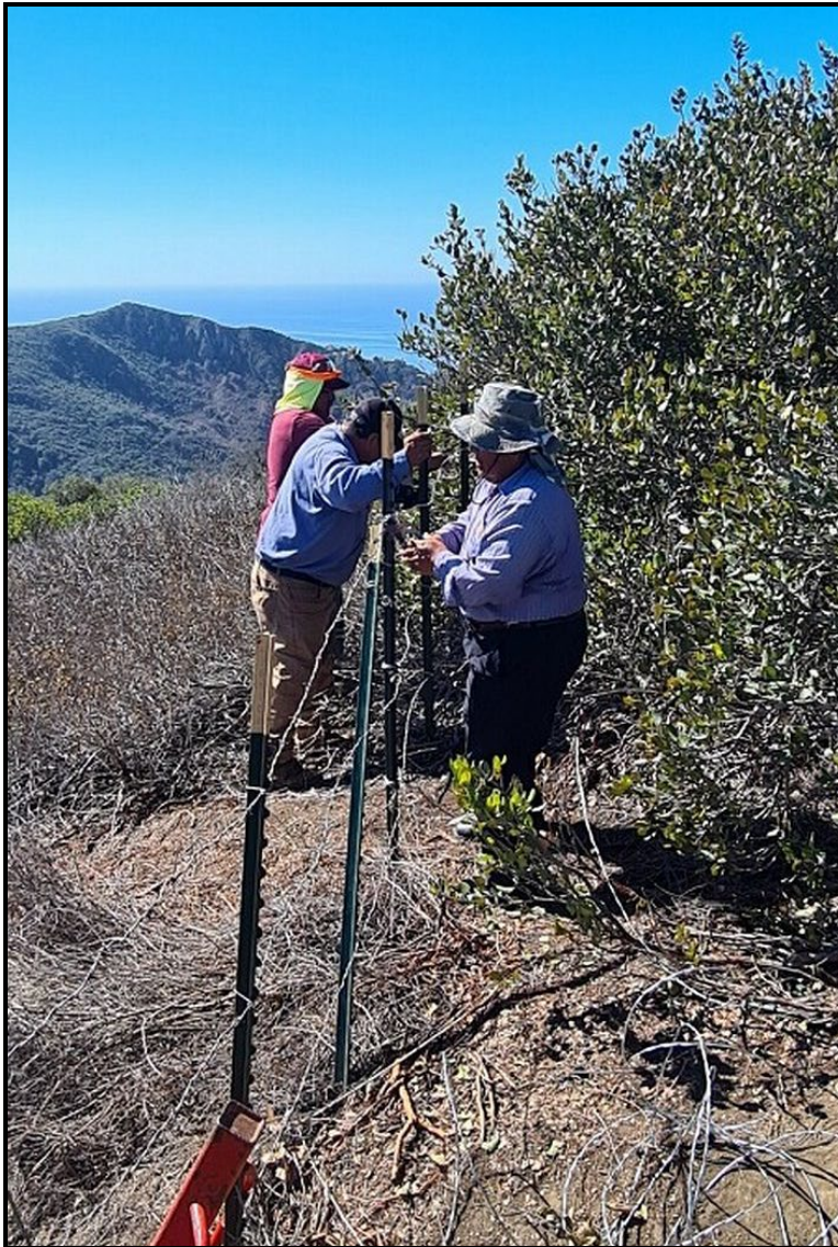
PHOTOGRAPH 32 Repaired Damaged Fence on Decommissioned Trail Leading to Burned Area at Pacific Horizon Preserve, September 2022
