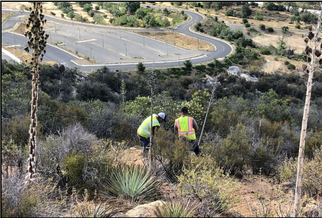
PHOTOGRAPH 21 Repairs to Damaged Fence Along Eastern Boundary of Silverado Chaparral Preserve, June 2022
