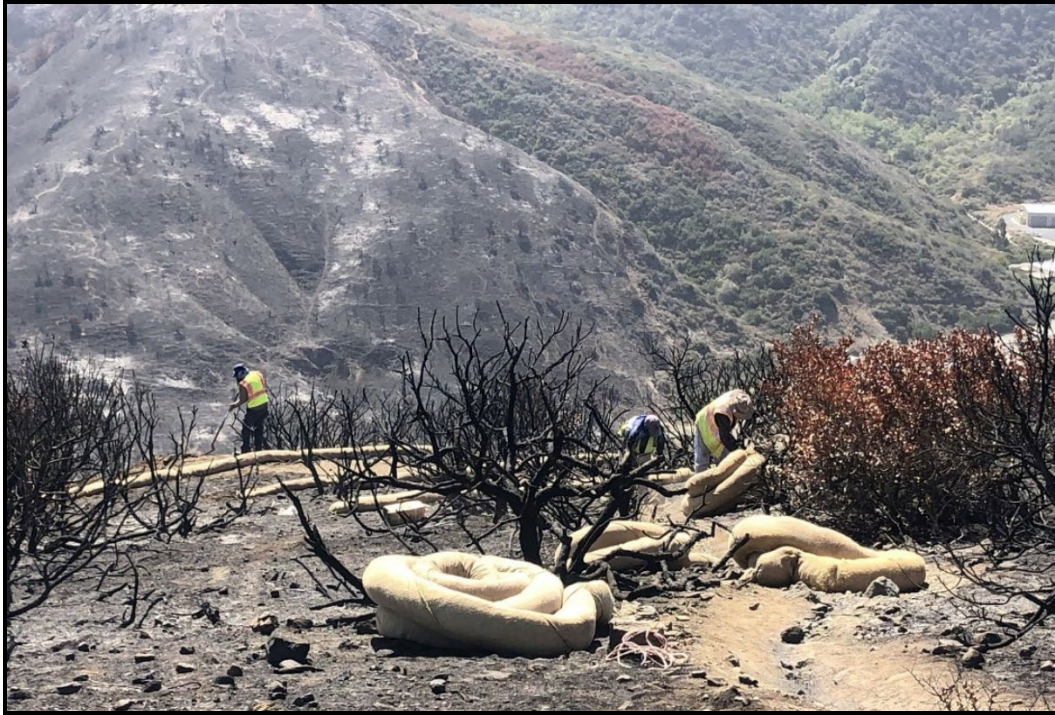
PHOTOGRAPH 28 Installation of Biodegradable Fiber Rolls in Burned Area of Pacific Horizon Preserve, June 2022
