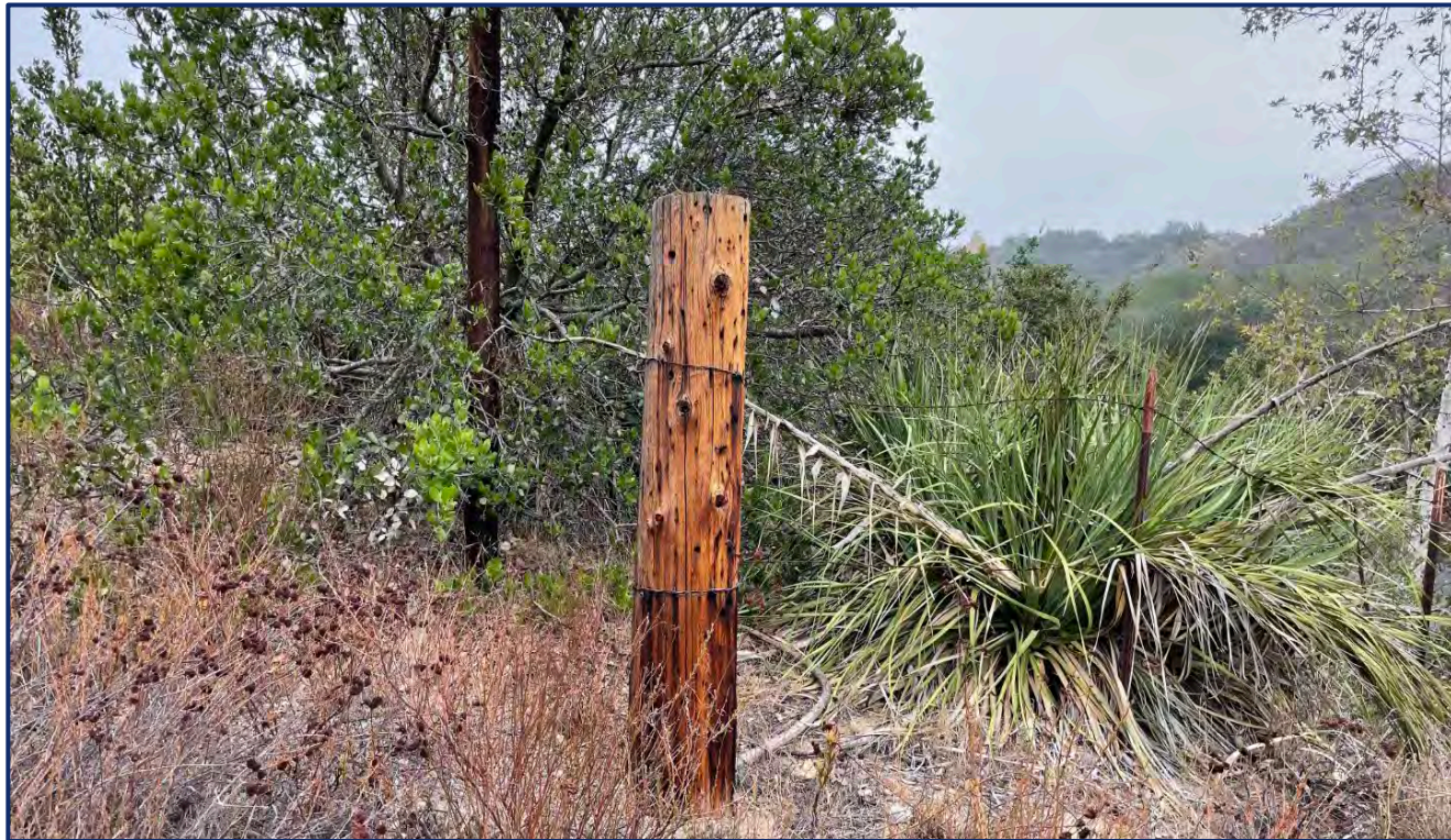
Photograph 3: Depicting area in need of fence repair. Photo taken October 13, 2022.
