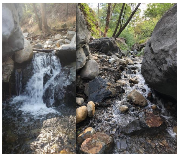
USFS Dam Restoration Project – Dam 8 Before and after removal (photo courtesy of USFS)
