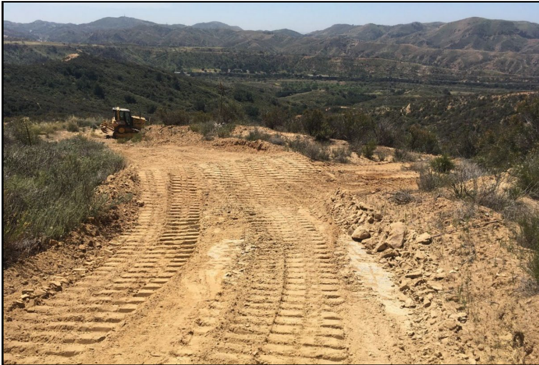
PHOTOGRAPH 18 Recontouring of Fire Road with Heavy Equipment to Fix Erosion at Silverado Chaparral Preserve, April 2022
